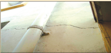
External Wall Cracks
